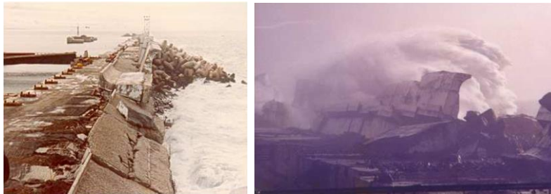
Sines breakwater failure, 1978/9
